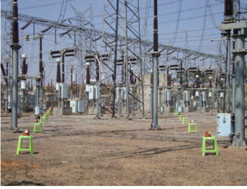
Fig. 3. A view of the 440 KV power distribution yard, showing the layout of equipment; apart from the transmission towers, several transformers and a firewall can be seen at a distance.
